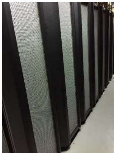
RDHx's – Typical Installation
