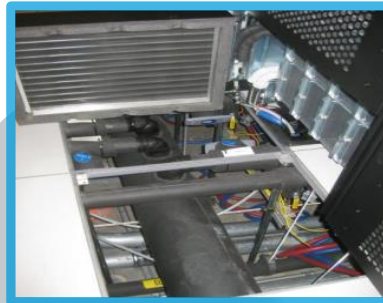
RDHx and Piping
